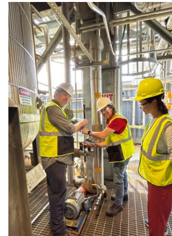
NETL fiber optic amine degradation sensor assembly and installation at NCCC
